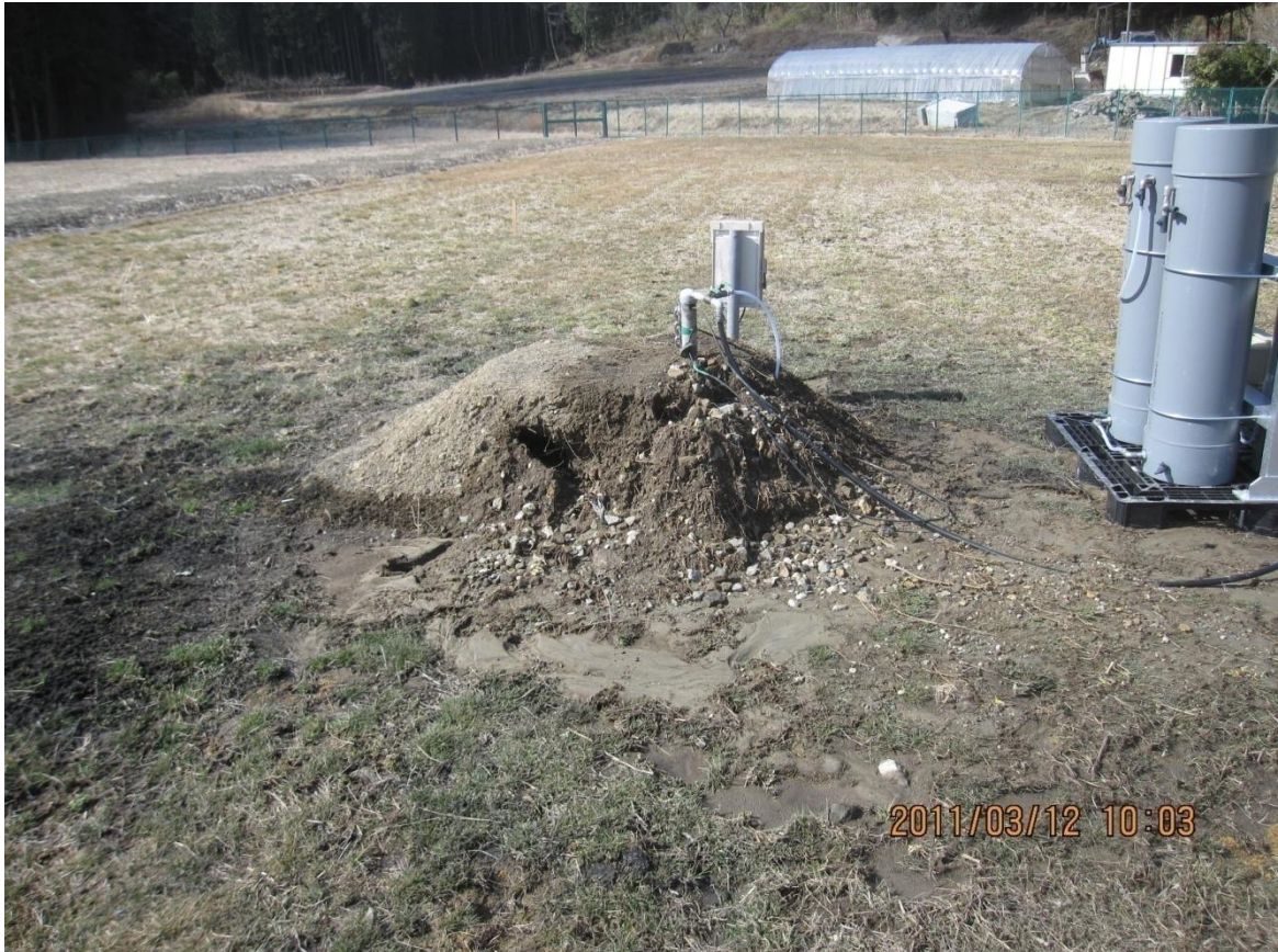
③-1 No. 3 浸透水噴出跡
